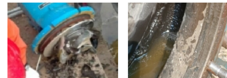
Secondary sludge intermediate reuse water pump P103026A at Huazhong (no ultrasonic)
