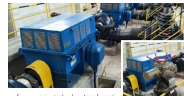
Energy-saving technology transformation of the circulating water system at the thermal power plant of Shanying Huanan
