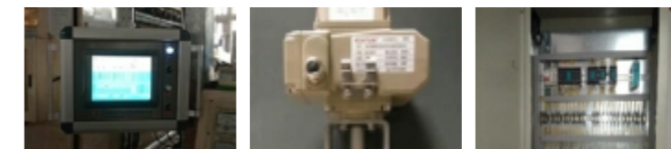
General control interface
